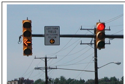
Photo of existing flashing yellow installation in the City of Alexandria, VA.
